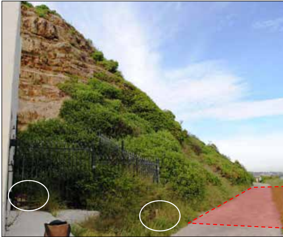
Figure 1 Geo-hazard #1 – Rock fall(s) into vegetation, existing fence or onto Nobby’s breakwater shared pathway. Pathway rock fall risk area shown in red. Past rock falls circled.
