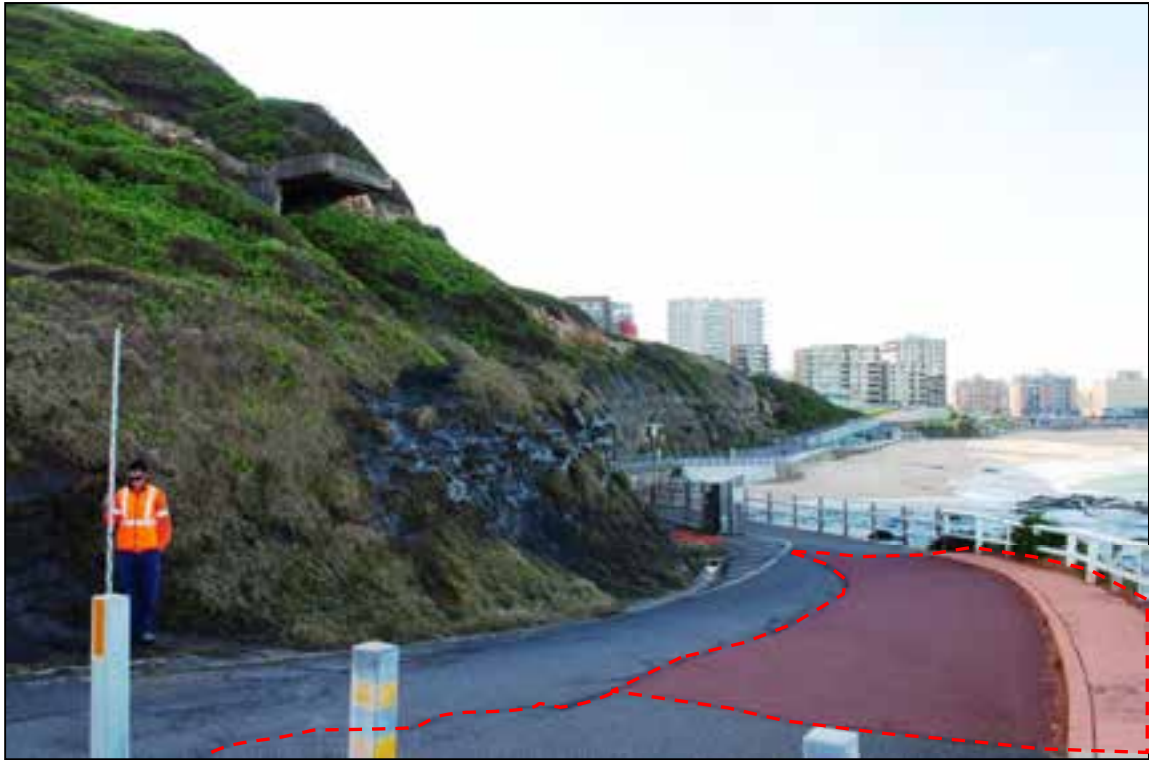
Figure 11 Geo-hazard #10 – Tension crack & settlement of coastal edge of Shortland Esplanade, shown in red. Hazard associated with deep fill supported by an old mortar block retaining wall.
