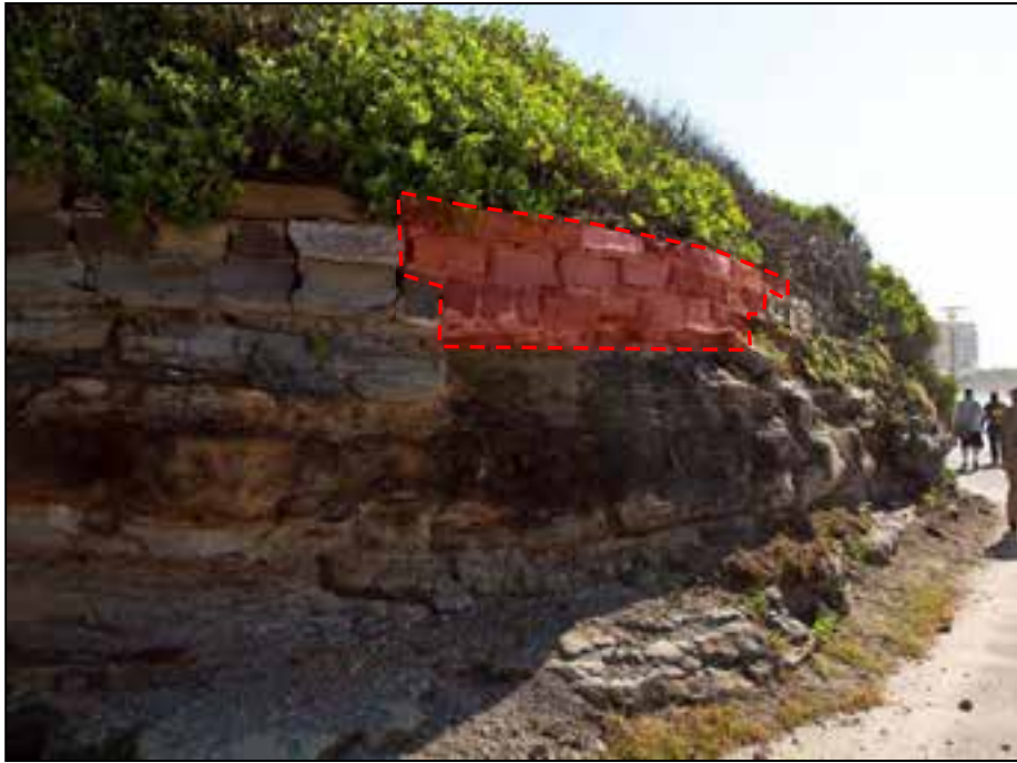
Figure 7 Geo-hazard #6 – Unsupported section of block wall (shown in red) falls onto Newcastle Beach footpath. At a meeting on 23/3/2012 CoN reported this section of wall had failed.
