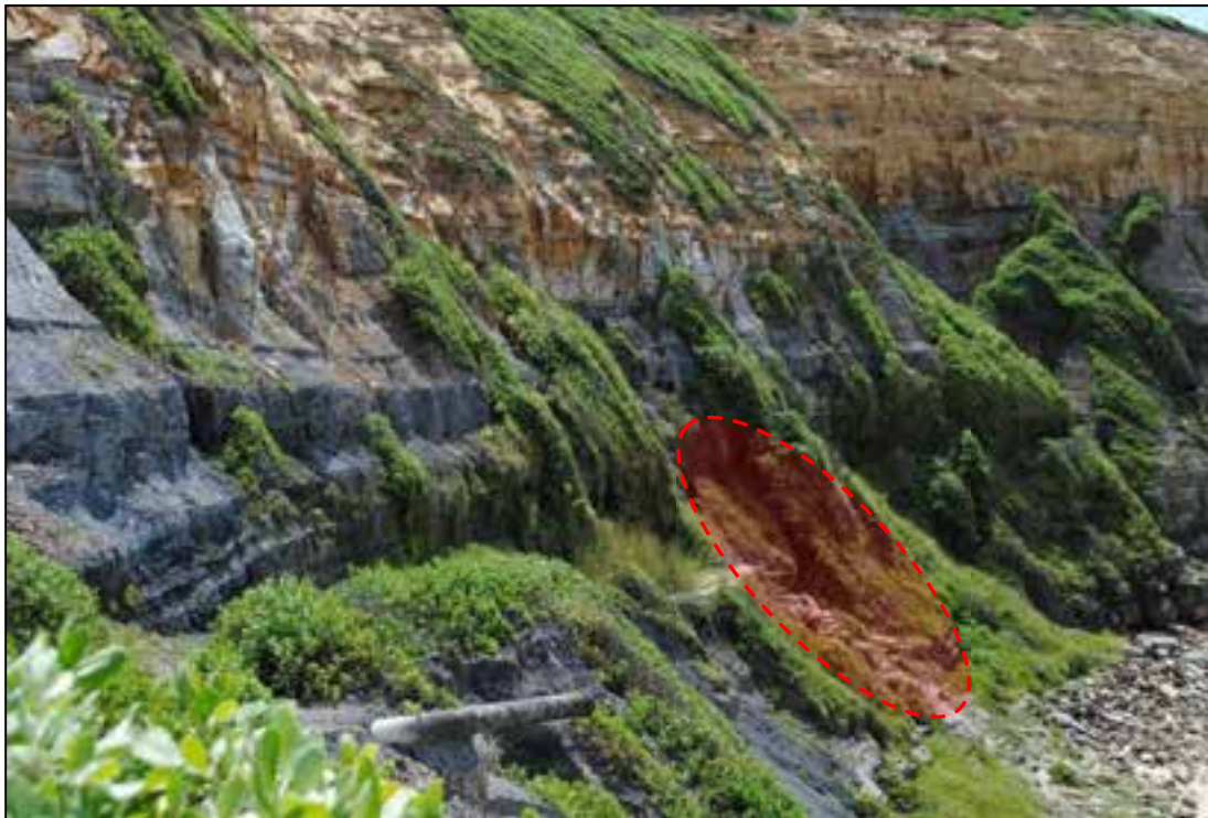
Geo-hazard #15 – Landslide failure in May 2001 destroyed hillside staircase to Susan Gilmore Beach, circled.
