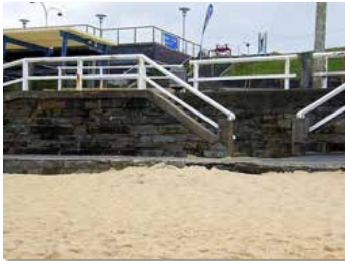
Plate 2.9. There are a variety of retaining structures along Bar Beach, of unknown construction. The walls behind the promenade and up the slope to the road above are unlikely to be designed for any sort of wave loadings. Photo: Coastal Environment 30/04/2011.
