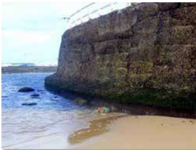
Plate 2.15. Exposed section of the seawall at the south end of Nobbys Beach suggests a construction of stone blocks, possibly with a later addition of render. A substantial toe section can be seen and appears to be founded on the rock shelf. Photo: Coastal Environment 30/04/2011.
