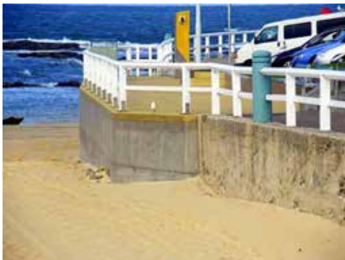
Plate 2.16. South of the SLSC and shelter shed, the roadway has been widened and a section of reinforced concrete seawall constructed. Photo: Coastal Environment 30/04/2011.
