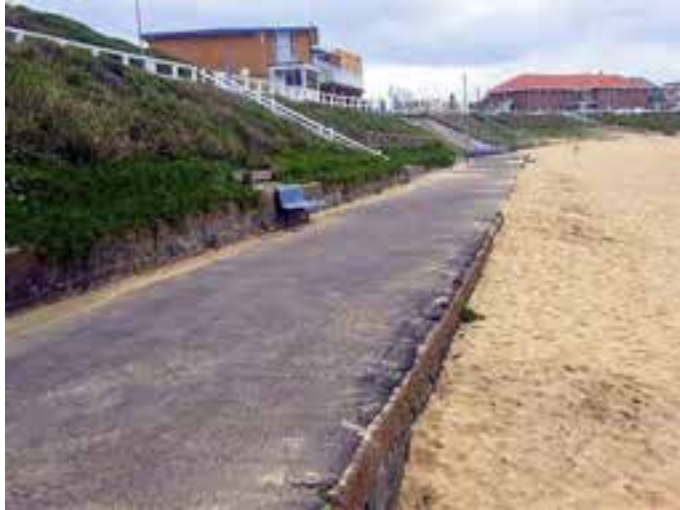
Plate 2.3 Walkway between Surf House and the SLSC, following the route of the old colliery railway line. There is a low vertical wall on the seaward side of unknown construction which is regularly overtopped by storm waves at present. This section of the beach appears to be shallowly underlain by bedrock. Photo: Coastal Environment 30/04/2011
