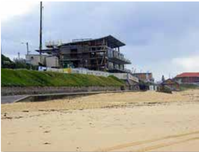
Plate 2.1 New Surf House at Merewether under construction. A mixture of high level and low level walls are constructed on the lower beach. The front pathway appears to follow the alignment of the old railway. Sections of the retaining structures, paving and fittings are in poor condition. Photo: Coastal Environment 30/04/2011
