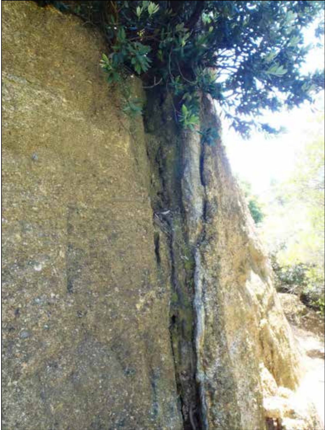
Figure 23 Geo-hazard #22 – Rock falls from south face of Obelisk Hill, due to tree root ‘jacking’ open and weathering of joints, as shown above. Observed rock falls have all come to rest within 3m of face.
