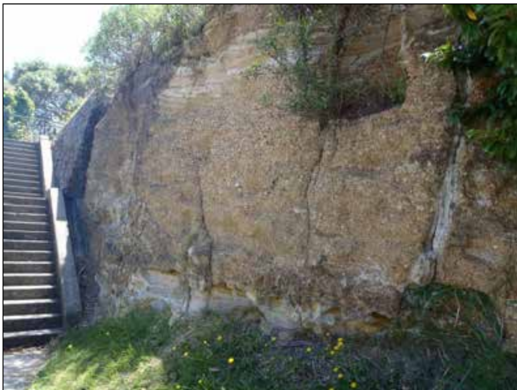
Figure 21 Geo-hazard #20 – close up of rock face & stairs, shows rock mass defects and vegetation growing in rock defects. Tree roots in rock face defects appear to be the cause of most rock falls. Observed rock fall blocks mostly \leq 300\text{mm} in diameter and have come to rest within 2m of cliff face
