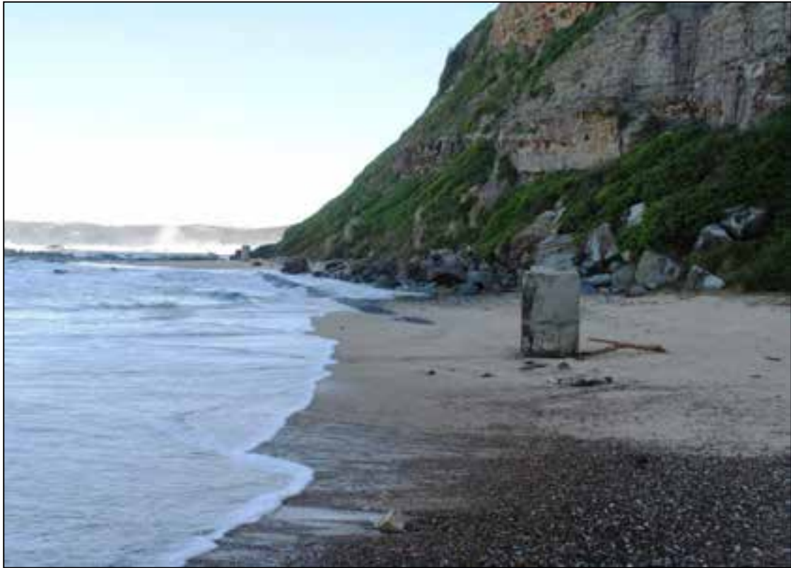
Figure 7 HWC Sewer inundated at sea levels approximating BMT WBM modelled year 2100 mean sea level – some vents at sea level allow pipeline to be flooded with sea water.
