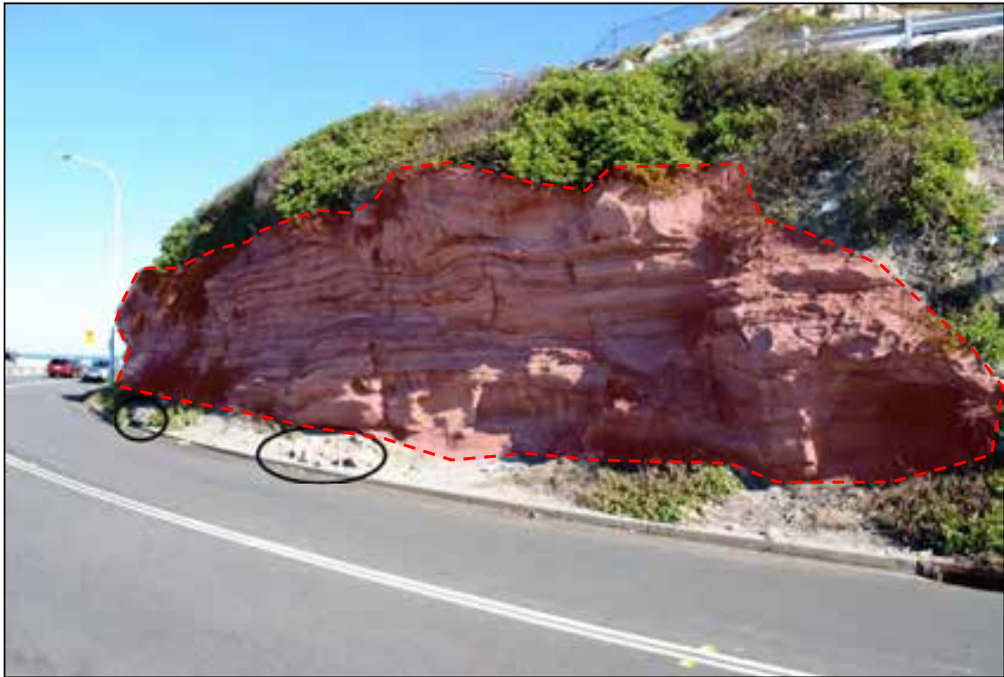
Figure 4 Geo-hazard #4a – Rock fall(s) onto Shortland Esplanade, hazard area outlined in red. Past rock fall debris, circled in black. Historical photos show rock debris on road.
