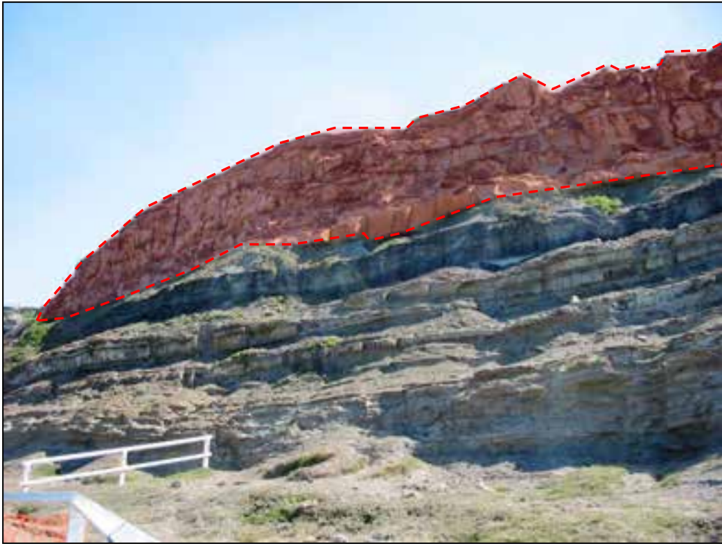
Geo-hazard #12a –Rock falls from cliff above Bogie Hole viewing area, due to erosion & weathering along open joints in a blocky sandstone unit, shown in red. This cliff/slope was ‘groomed’ after 2003 rock fall.
