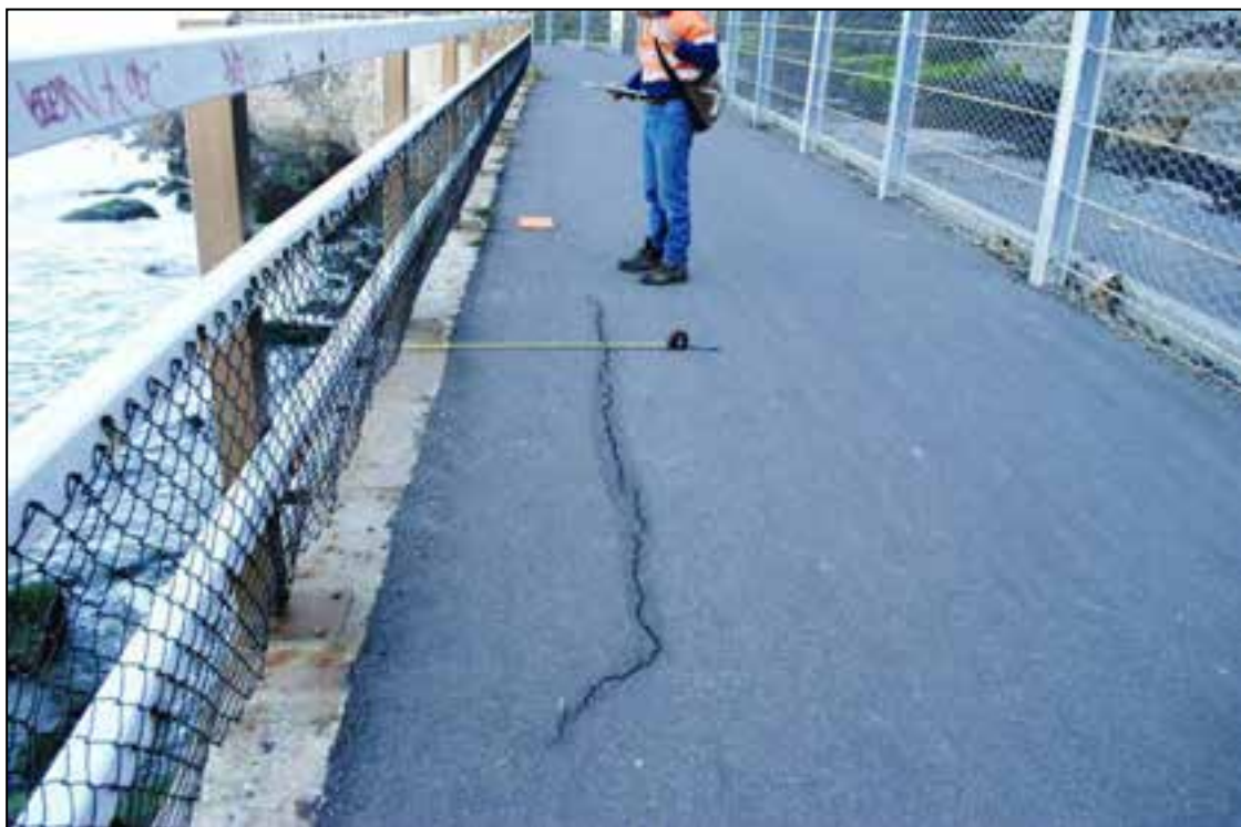
Figure 10 Geo-hazard #9– Tension crack/ differential settlement in recently sealed walkway. Hazard associated with deep fill behind sea wall at South Newcastle.
