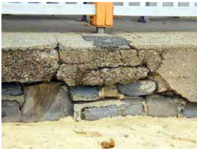
Plate 2.4. Low retaining /seawall seaward of the shelter sheds. The original wall is of stone blocks with mortar that is eroding. Concrete paving has been poured over this and is cracking. Much of this structure is in poor condition and could be further damaged under wave action. Photo: Coastal Environment 30/04/2011
