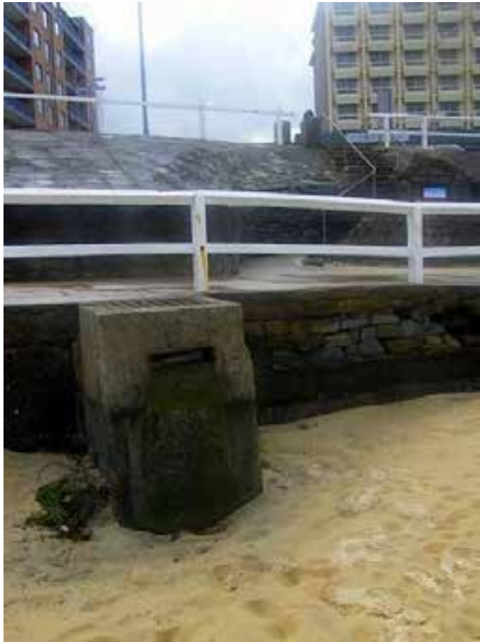
Plate 2.13. At Newcastle Beach there are a range of protection structures at a low level separating the walkways, change sheds and paved areas from the sandy beach. These are of variable quality and largely undocumented construct. Stormwater services are intertwined with the protection works. Photo: Coastal Environment 30/04/2011.
