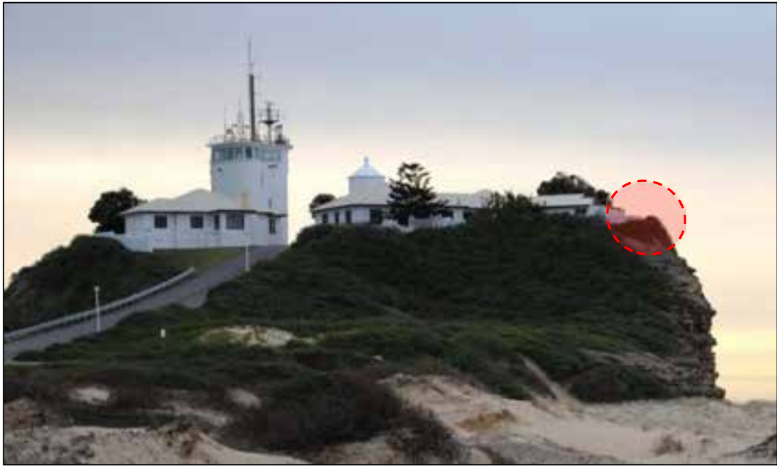
Figure 3 Geo-hazard #3 – Cliff top regression encroaching into existing development on the south side of Nobby’s Headland. At risk structures (hi-lighted in red) are setback less than 3-5m from crest of weathering cliff face, with one corner of boundary fence ‘suspended’ over steep slope.
