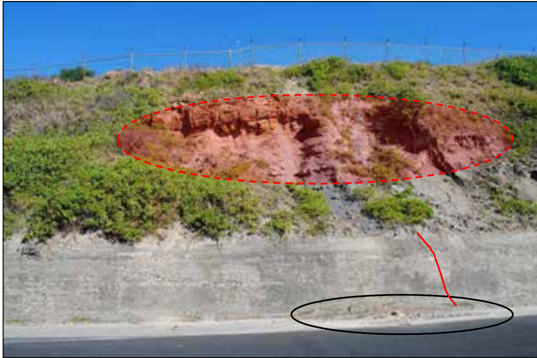
Figure 5 Geo-hazard #4b – Rock fall(s) from blocky outcrop (shown in red) onto Fort Drive. Past sediment and rock falls circled. Note, crack (red line) in concrete wall; cracks were observed at several other locations along this wall.
