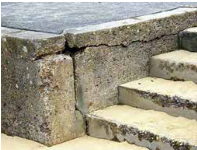
Plate 2.2. Stairs leading from the walkway to the beach. Construction details are not known. The front seawall of vertical concrete construction is exposed to wave action and has rotated seaward at the top with cracking extending through the structure. Photo Source: Coastal Environment 30/04/2011
