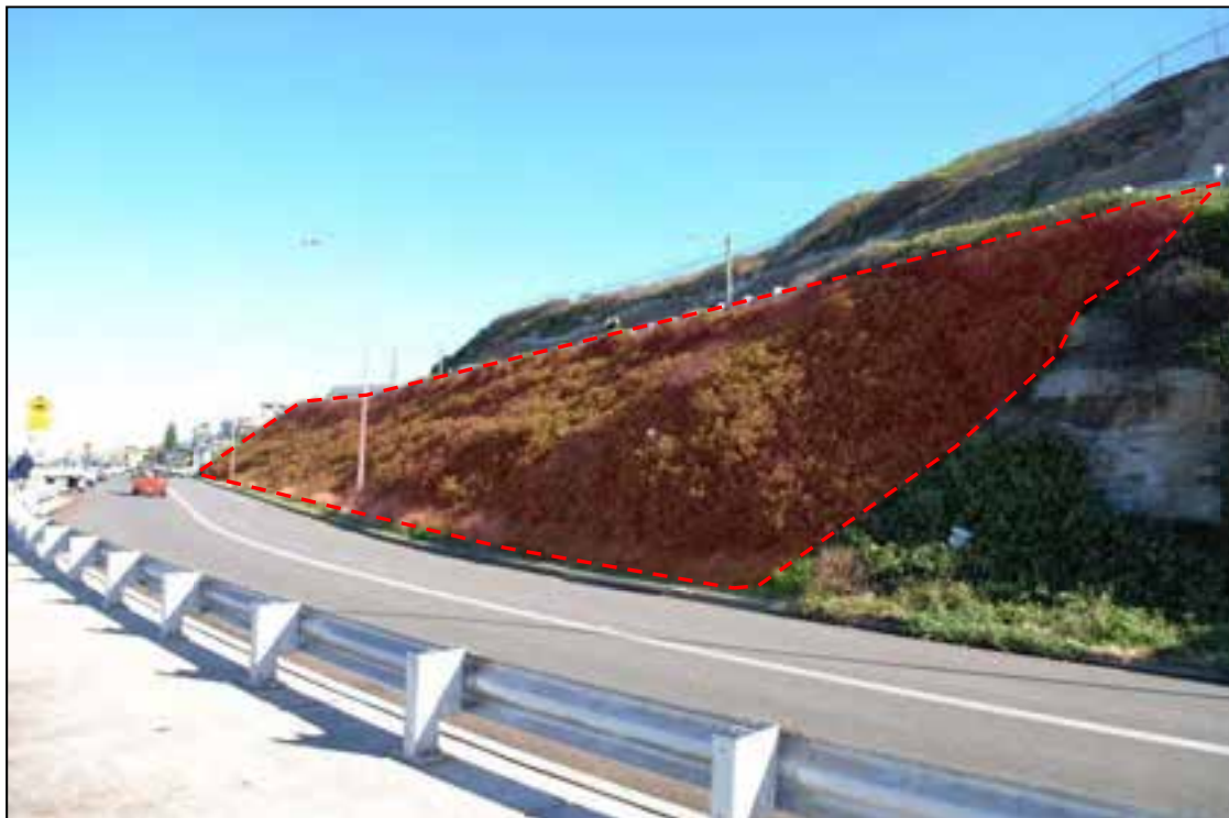
Figure 6 Geo-hazard #5 – Vegetation covered fill batter/ shallow soil slope above road, shown in red. Potential for shallow failure of mixed debris onto Shortland Esplanade.
