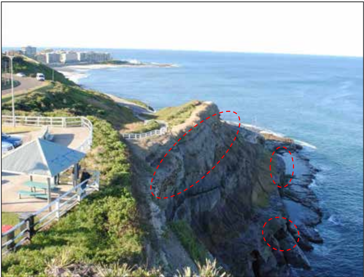
Figure 5c Cliff/slope above Bogey Hole: 1896, 1998 & 2011 looking north. Areas of apparent cliff line regression circled.
