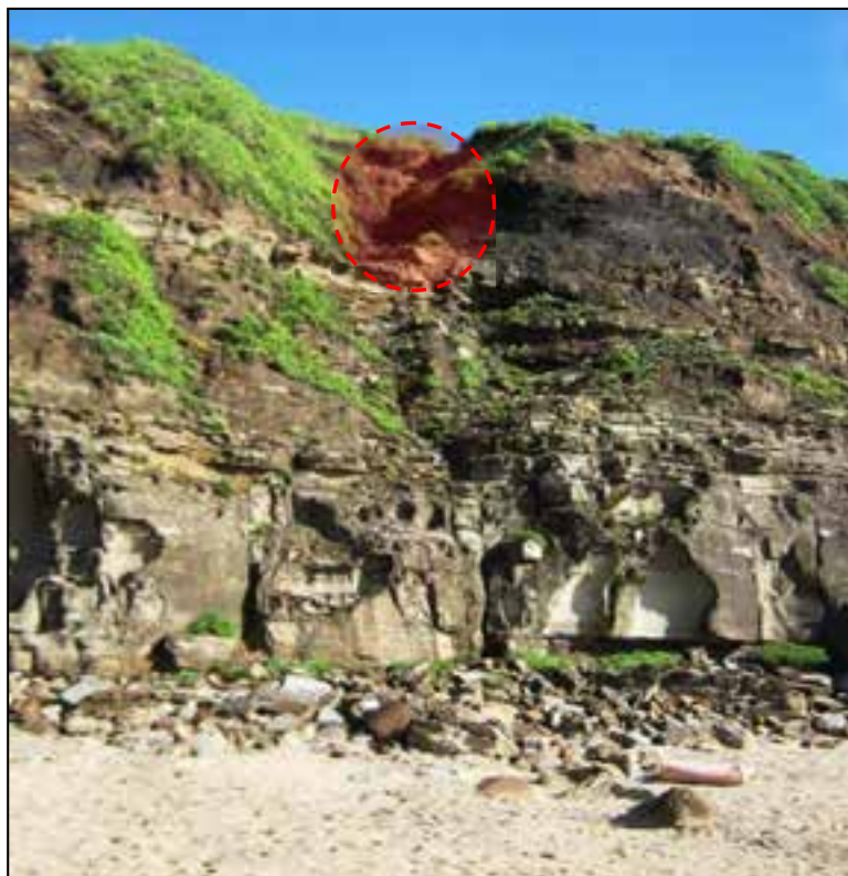
Figure 16 Geo-hazard #15 – Cliff / slope deeply scoured by stormwater discharge onto upper and mid-slope areas. Soil/ extremely weathered rock and Dudley Seam almost completely eroded in circled area by stormwater discharge.
