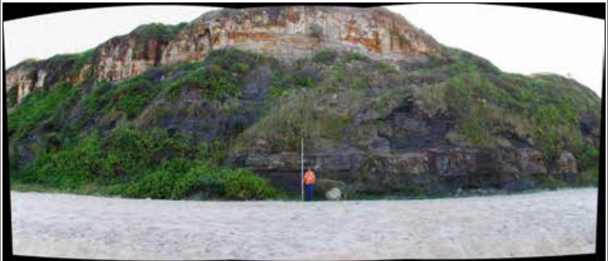
Figure 18 Geo-hazard #17– ‘The Cliff’ below Kilgour Avenue, past slide(s) debris and rock falls cover/ litter beach at toe of cliff/slope. Past instability has been associated with intense rainfall events and has resulted in sections of the beach being closed whilst slope stability has been re-assessed.
