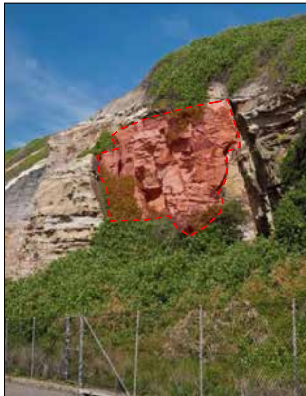
Figure 8 Geo-hazard#7 – Massive block(s) fall risk, shown in red. Rock fall analysis indicates it is unlikely to reach fence.
