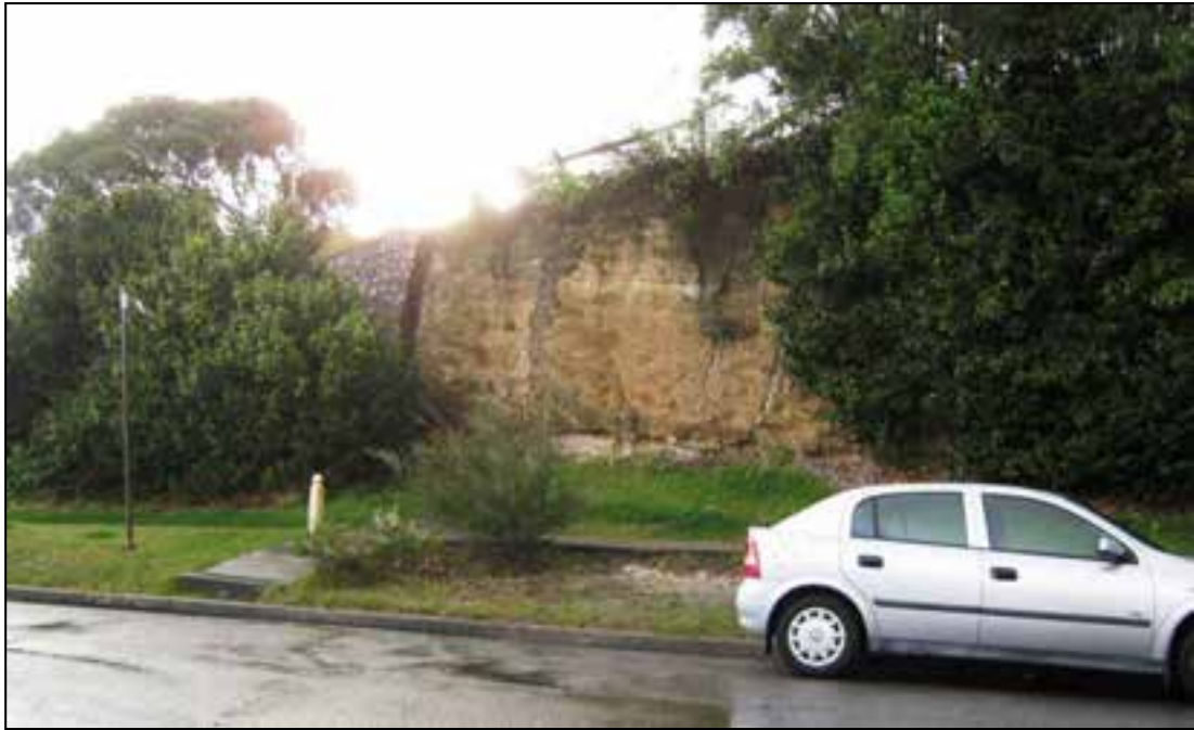
Geo-hazard #20 – Rock fall(s) from Obelisk cliff face onto pedestrian footpath.
