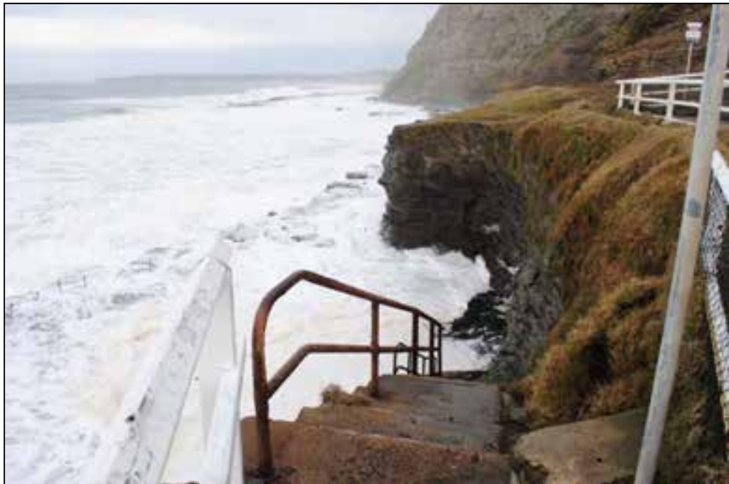
Figure 13 Geo-hazard #12b – Increased frequency of rock falls due to increased wave attack on sea cliff adjacent to Bogie Hole rock platform. (Photo shows storm swells approximately 1¾ hours past a 1.3m high tide. Wave set up approximates BMT WBM modelled year 2100 mean sea level)
