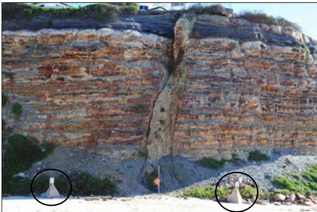
Figure 2 Geo-hazard #2 – rock fall(s) from cliff face onto beach. Warning signage (circled) provides visual warning; however ~ 10% of rock blocks have ‘run out’ past signs.
