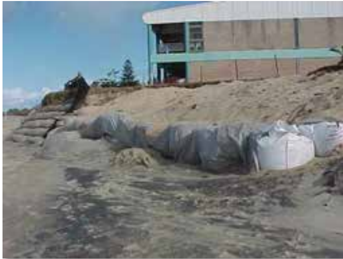
Plate 2.18. A temporary geotextile sand filled container wall was constructed in 1996 to protect the Stockton Surf Club building. This has recently been upgraded and extended further north. There are no formal protection works between the Surf Club and the Mitchell St. seawall. Photo: BMT WBM 26/07/1999.
