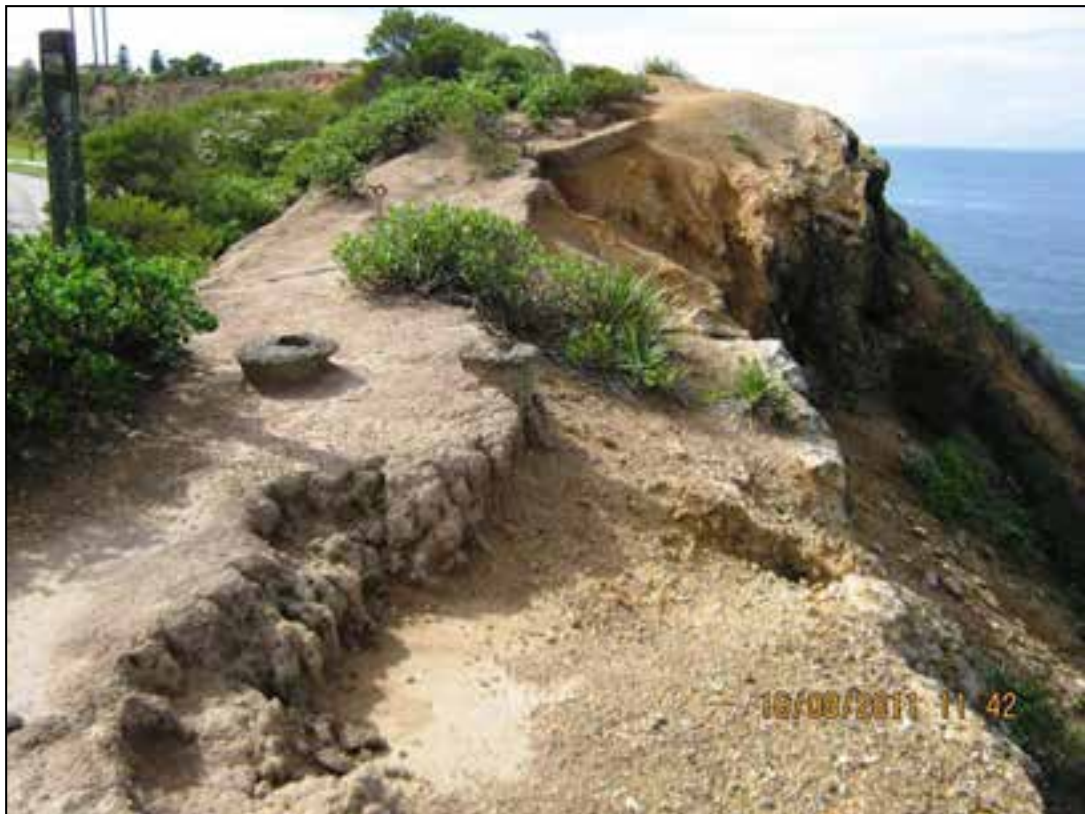
Figure 14 Geo-hazard #13 – Cliff top erosion resulting in ‘necking’ of cliff top from Strzelecki Lookout to Shepherds Hill along the proposed alignment of the Memorial Walk.
