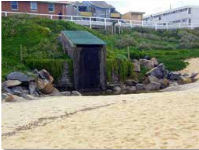
Plate 2.6. Stormwater outlet north of Watkins Street. Rock has been placed to protect the outlet structure which intersects the buried seawall
