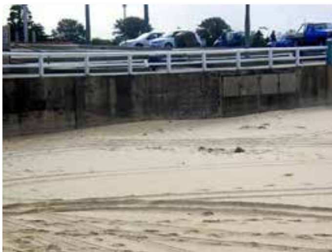
Plate 2.17. Along the northern section of Nobbys Beach there is a vertical seawall adjacent to the carpark. Construction details are unknown. The whole of Nobbys Beach to the north is backed by the early 19th century construction of Macquarie Pier joining Nobbys Head to the mainland. Photo: Coastal Environment 30/04/2011.
