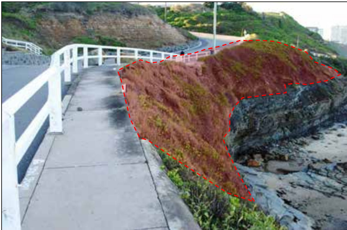
Figure 12 Geo-hazard #11 - Creep movement of Shortland Esplanade fill embankment, shown in red, has resulted in stepped/ cracked pavement. Fill embankment creep & instability and sea cliff regression has resulted in loss of access to concrete footpath.
