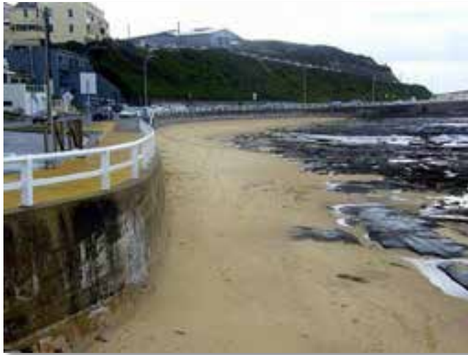
Plate 2.14. North of Newcastle baths, the old near vertical seawall continues along the shoreline to Nobbys Head. Again this seawall appears to be constructed on the rock shelf along Shortland Esplanade. Construction and foundation details are unknown. Photo: Coastal Environment 30/04/2011.
