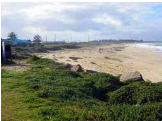
Plate 2.20. North of the end of the Mitchell St seawall at Stone St., there is no protection of the back beach area which has eroded into the dune fronting the child care centre and further north. Photo: Coastal Environment 30/04/2011.
